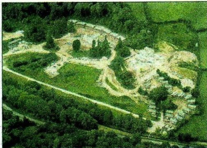
A bird's-eye view of The Cornwall Hotel Spa and Estate in St Austell.
